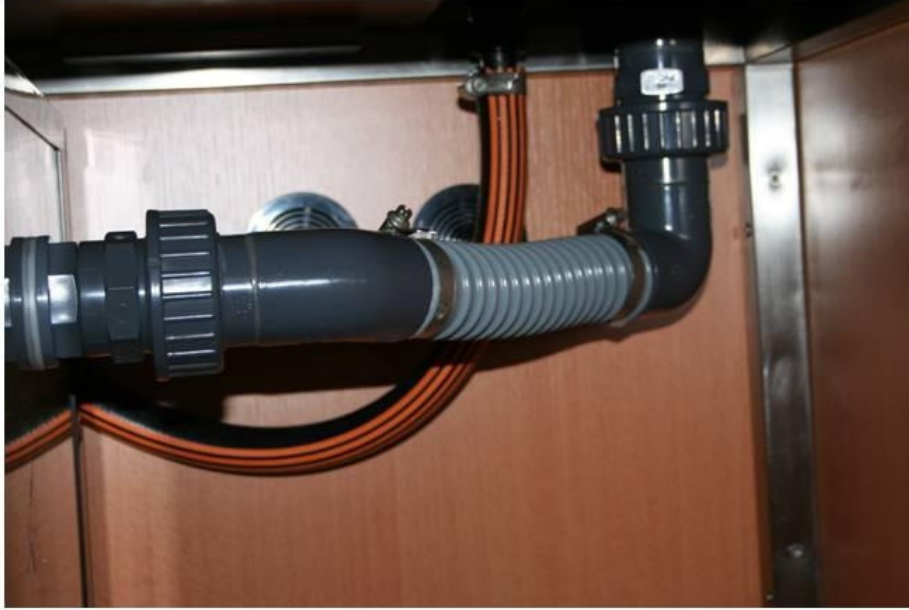
Fig. 2: Drainage fittings installed. The striped pipe behind is the flexible hose that connects the Ocean Runner 3500 to the hositail on the bottom of the 25 mm rigid pipework tank connector.
